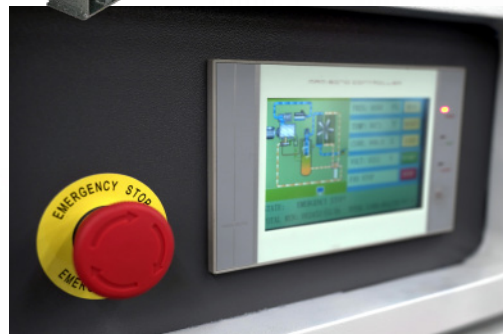
Digital Control Panel
